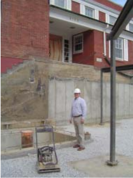
The picture is from the new lower level . . . the elevator is to the right of Jim Mann and above his head is the old entry from the south parking lot.
