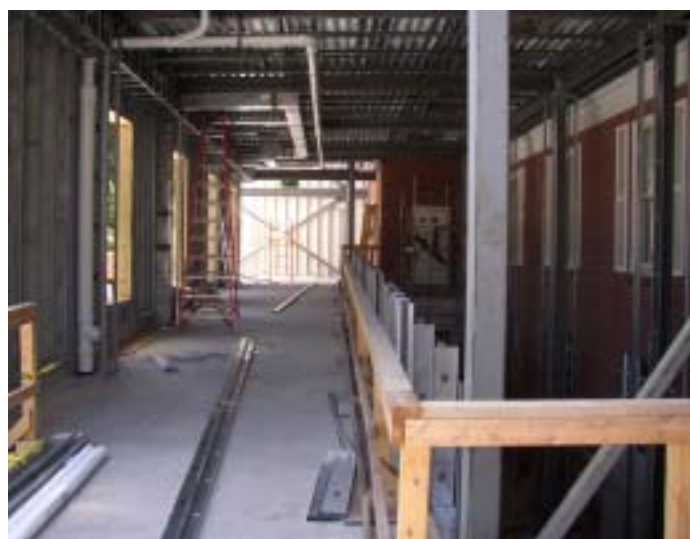
Looking up the new ramp from the Gathering Space to the sanctuary
